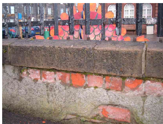
Figure 12e: Physical weathering of a school wall, plus chemical weathering of a railing
