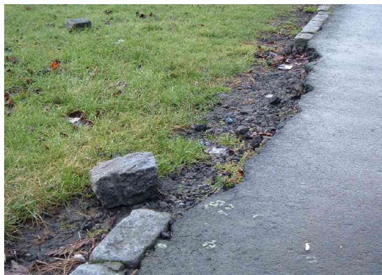
Figure 12a: Physical weathering of the edge of a path. Many of the kerbstones have been removed by 'erosion'.
