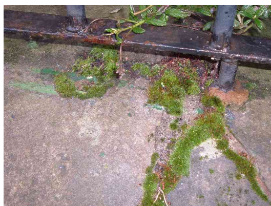
Figure 12f: Biological weathering by moss growing in cracks
