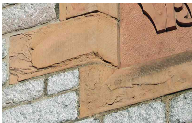
Figure 12d: Different building stones weather at different rates: granite is more robust than sandstone
